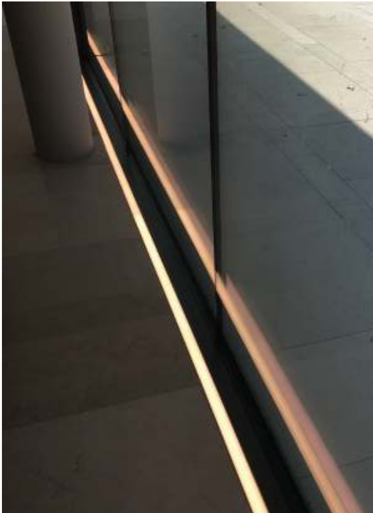
LED verlichting langs glazen pui in de foyer
